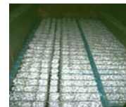
COD treatment - Biological system
