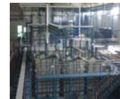
General Metal and COD treatment system
