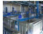
COD treatment - Fenton System
