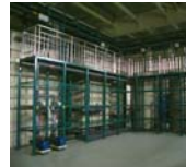
Spent waste Pre-treatment system
