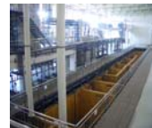
Wastewater collection tanks with leaking detection & containment
